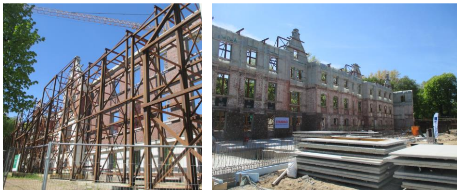
Figure 4 and 5: Photos of the construction site at the laying of the foundation stone in May 2017 (Photos: I. M. Reuther).
